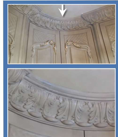
On site completed project showing the curved Acanthus Crown Molding sections installed.
